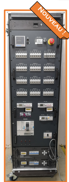
SRS Armoire de distribution 400A
